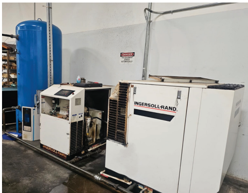
Ingersoll-Rand SSR-EP155E Rotary Screw Air Compressor, 56CFM, 125PSIG, 15HP, s/n KE0249U94227, w/ Vertical Air Tank and Air Dyrer
