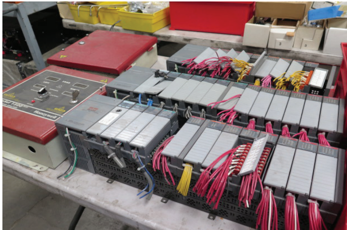
Allen Bradley PLC Components
