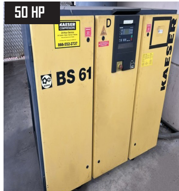
Kaeser BS-61, 50 HP Rotary Air Compressor with Tank and Dryer.
