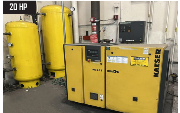
Kaeser AS-20T, 20 HP Rotary Air Compressor w/ Tank System.
