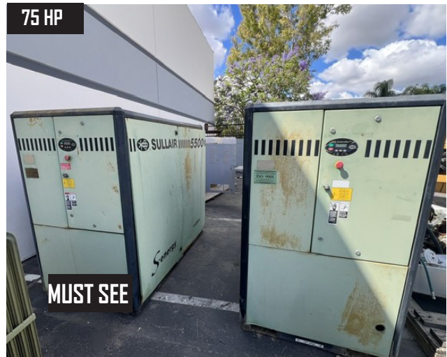
75 HP MUST SEE (2) Sullair 5507/A 75Hp Rotary Air Compressors w/ WS Digital Controls.
