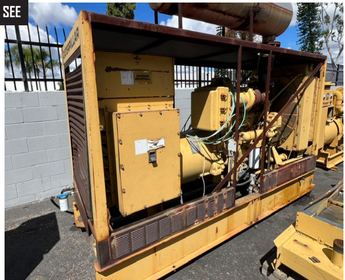
Caterpillar mdl. 3406 300kW STANDBY 240/240V Diesel Generator Set w/ Turbo Diesel Engine.
