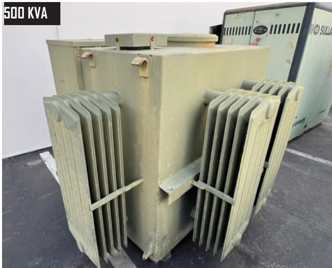
500 KVA Standard Transformer 500kVA Distribution Transformer 13,200 Delta Rated Voltage.
