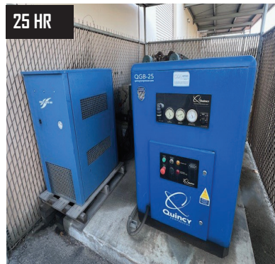
Quincy QGB-25 Rotary Air Compressor with Great Lakes Dryer.
