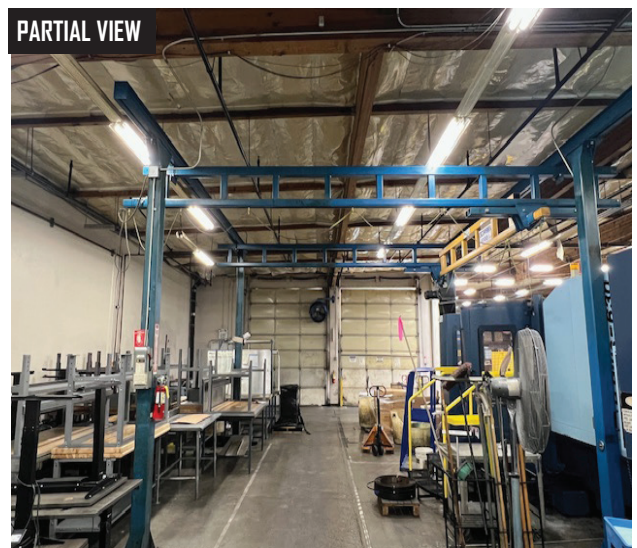
(One of Many) Gorbelt 4000 lb Capacity Crane System
