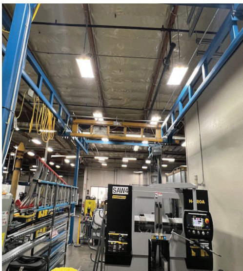
(One of Many) Gorbelt 4000 lb Capacity Crane System.
