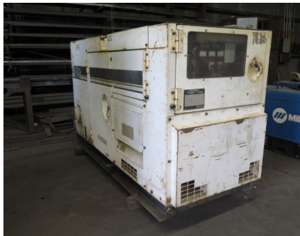
MQ Whisperwatt DCA44 SPX 44kVA Diesel Generator s/n 365-6809 w/ Isuzu 4-Cylinder Diesel Engine.
