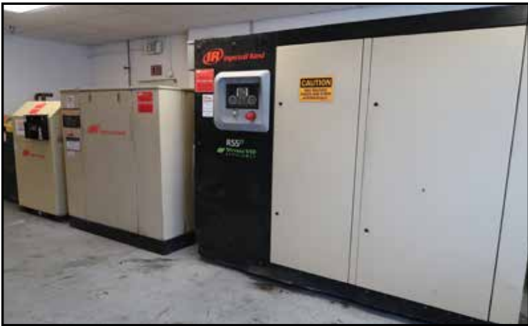
View of Ingersol Rand Rotary Air Compressors with Dryer
