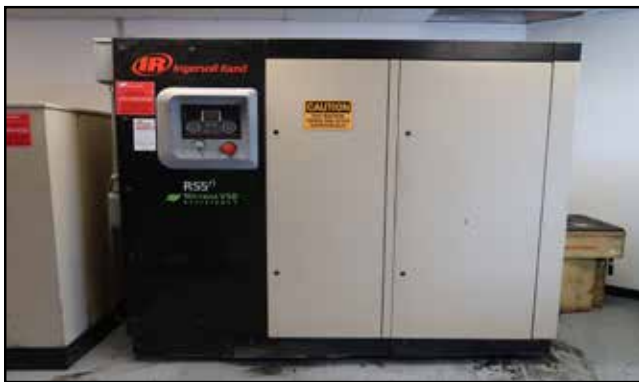
Ingersoll Rand R55N-A145 "Nirvana VSD Efficiency" 75Hp Rotary Air Compressor s/n NK1183U12103 w/ Ingersoll Rand Digital Controls.
