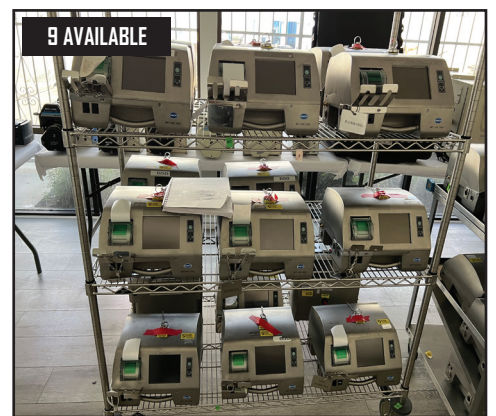
9) HATCH PARTICLE COUNTERS.
