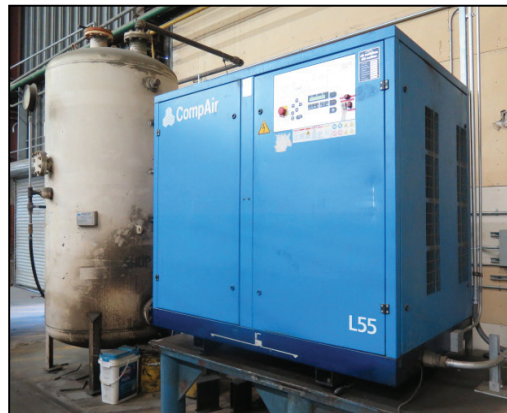
2002 Compare L55 75Hp Rotary Air Compressor
