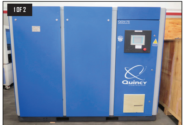
QG-75 75Hp Rotary Air Compressor w/ Siemens Simatic Touch Panel Controls
