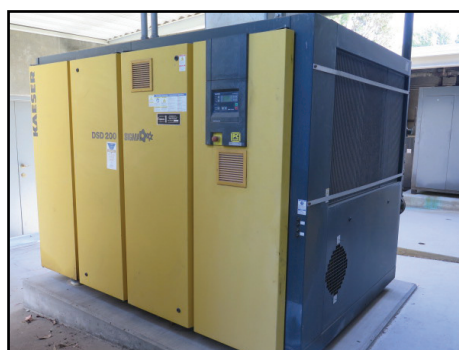
Kaeser DSD200 200Hp Rotary Air Compressor w/ Sigma Controls, 40,166 Run Hrs, 14,665 Load Hrs
