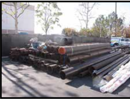
LARGE SELECTION OF PIPE MATERIAL
