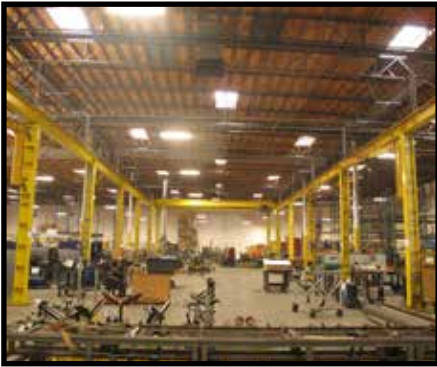
OMI 5 TON OVERHEAD SELF CONTAINED GANTRY UNIT, 5 GORBEL 1 TON JIB
