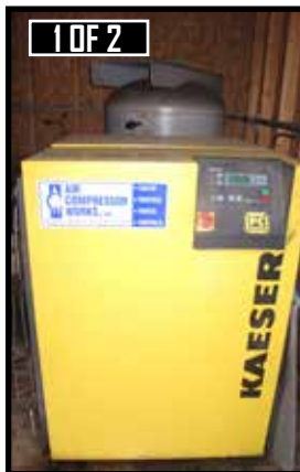
KAESER SK 26 ROTARY AIR COMPRESSOR W/ AIR DRYER. (1 OF 2)
