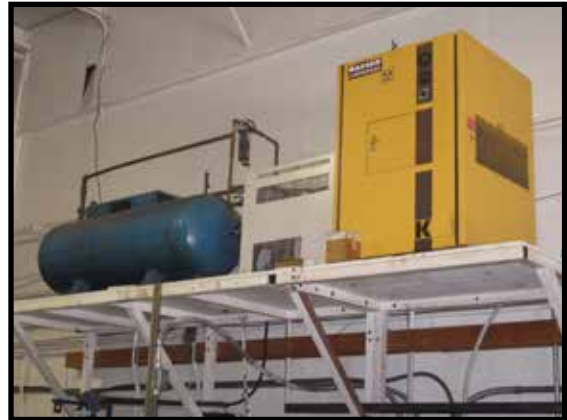
KAESER ROTARY AIR COMPRESSOR WITH DRYER AND TANK.
