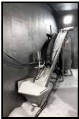
SAND BLAST EQUIPMENT WITH RECOVERY SYSTEM.
