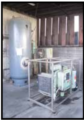
SULLAIR LS-10, ROTARY AIR COMPRESSOR WITH DRYER AND TANK
