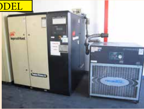
Ingersoll Rand IRN60H-CC 60Hp Rotary Air Compressor s/n NV2846U06195 w/ Intellisys Digital Controls, 145 Max PSIG.
