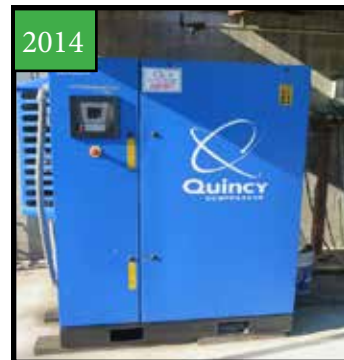
2014 QUINCY QGS40 40 HORSE ROTARY AIR COMPRESSOR
