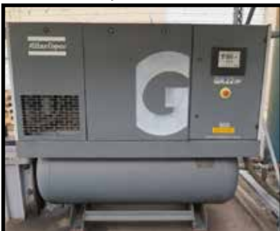
2007 Atlas Copco GA22FF Air Compressor
