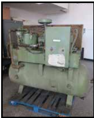
Joy Twistair 20Hp Rotary Air Compressor
