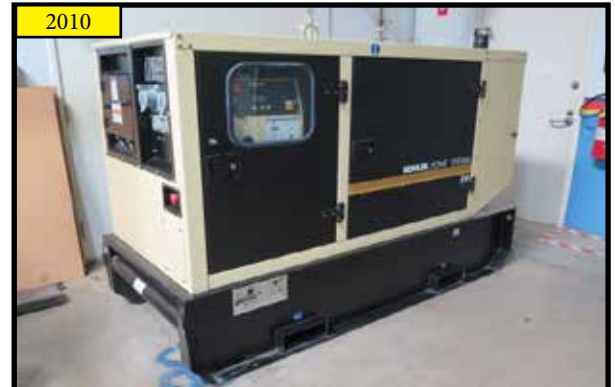
2010 Kohler Power Systems Type 20RE021 26kVA Diesel Generator
