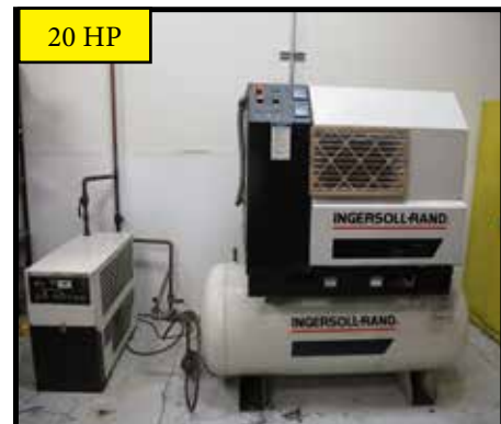
IR 20 HP ROTARY AIR COMPRESSOR, WITH DRYER AND TANK, MODEL SSR-EP20.
