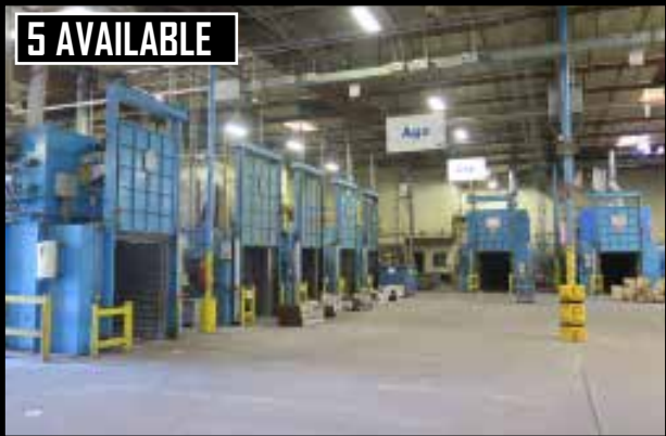
California Heating Equipment mdl. 4.5X30X4.5RT8 Artificial Aging Ovens
