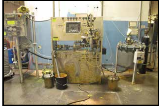
TRICO POLY SYSTEM POLYURETHANE PROCESSION LINE W/ CONTINOUS SLINGER DEGASSER, MKXX HYDRODESPENSER, BATCH MIXER.
