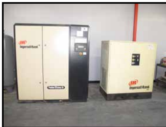
2003 Ingersoll Rand TMS0540 Refrigerated Air Dryer s/n TMS0540-0307/1354.
