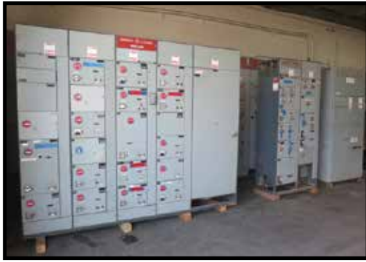
GE MOTOR CONTROL CENTERS
