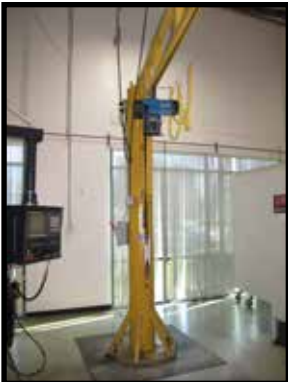
(1 OF 3) DEMAG 1000 LB CAPACITY JIB CRANE.
