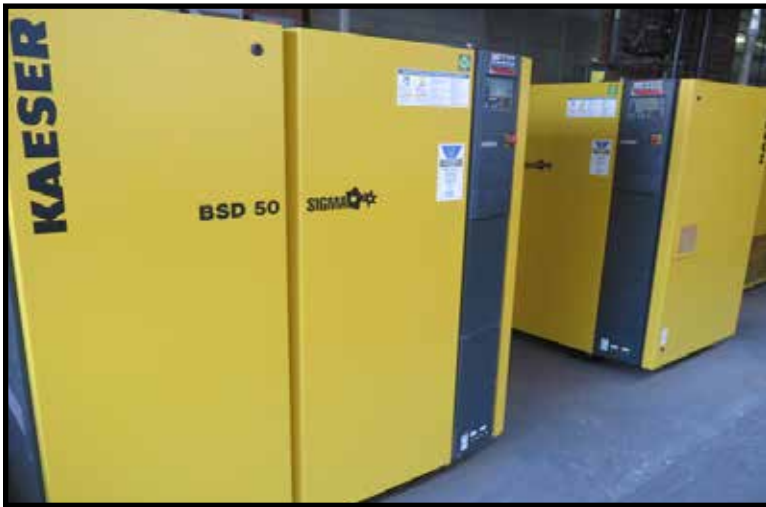
2016 Kaeser BSD50 Sigma 50Hp Rotary Air Compressors **2-AVAILABLE**
