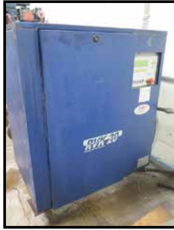
2007 Worldair RVK20 230/460V Rotary Air Compressor
