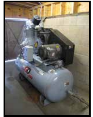
GARDNER DENVER 15HP AIR COMPRESSOR WITH DRYER.
