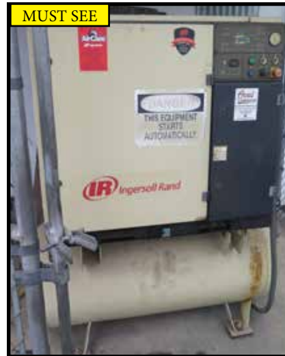
Ingersoll Rand SSR-UP6- 25-150 25Hp Rotary Air Compressor
