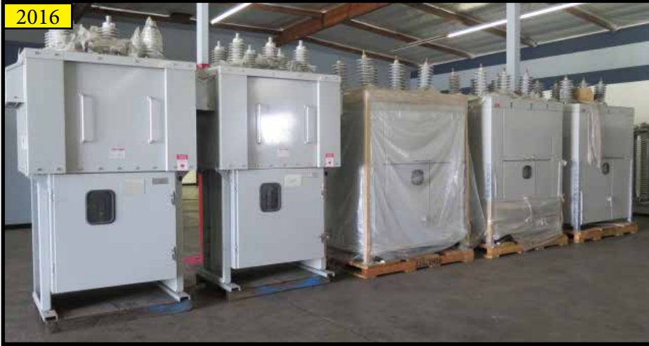
2016 ABB & Schneider Vacuum Substation Breakers
