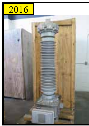
2016 GE Type OTCF-145EM Capacitor Voltage Transformers 145kV
