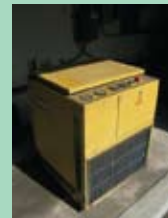
KAESER ROTARY AIR COMPRESSOR
